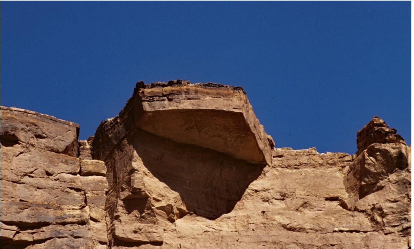
Fig 8.3 Here a large block has fallen and left a piece of its topmost part still attached weakly to the wall. With nothing supporting it, this rock could fall at any moment, most likely during heavy rain when water can penetrate and loosen whatever bonds still hold it on the wall. Campers noticing overhangs like this after they have set up may not sleep well.
